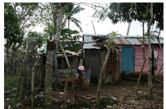
Storm-damaged houses in one of the areas Onè Respé works
